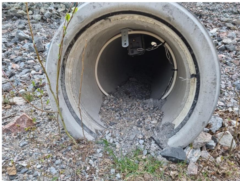
Figure 10 Picture of the camera positioned inside the ecoduct
